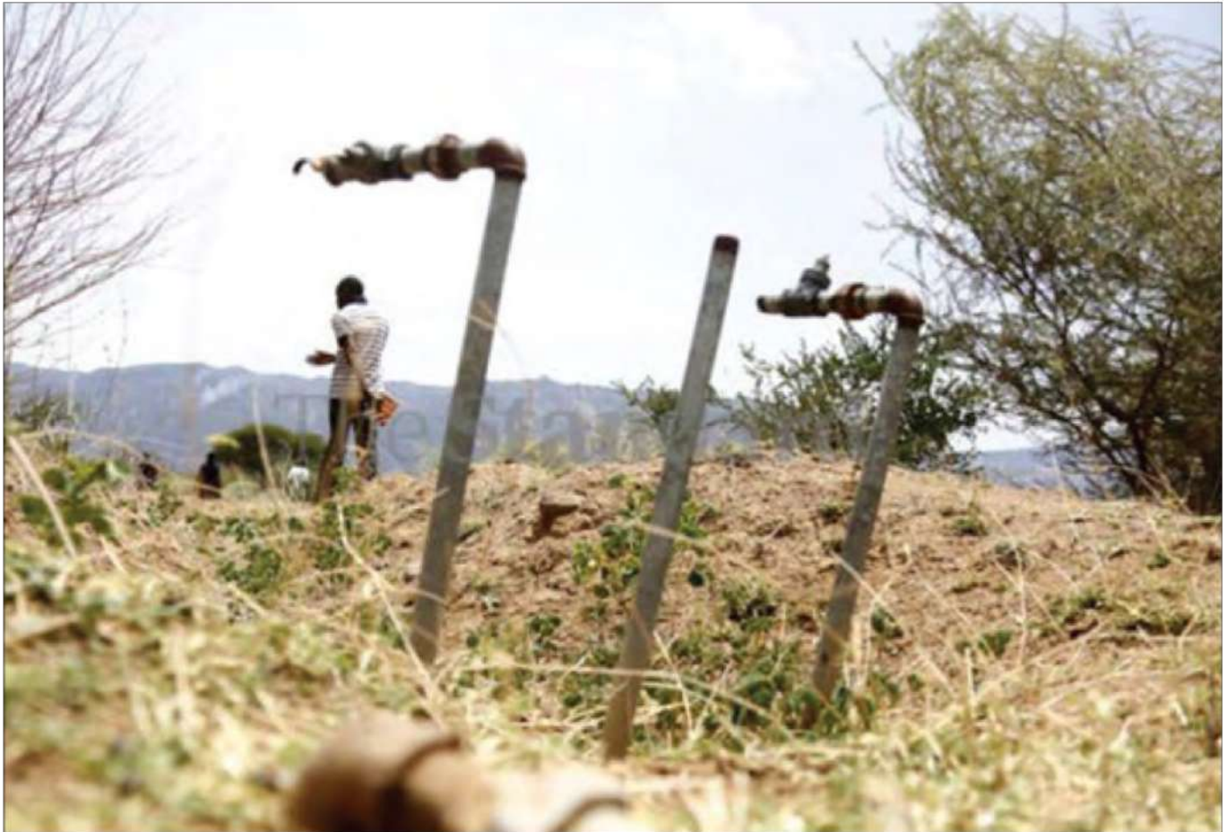
A vandalized irrigation pipe at Tot-Kolowa irrigation Scheme in Tiaty, Baringo county
